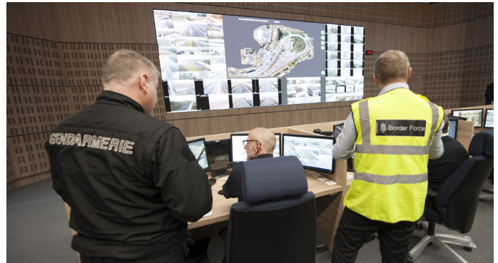
Eurotunnel Control Room Calais
